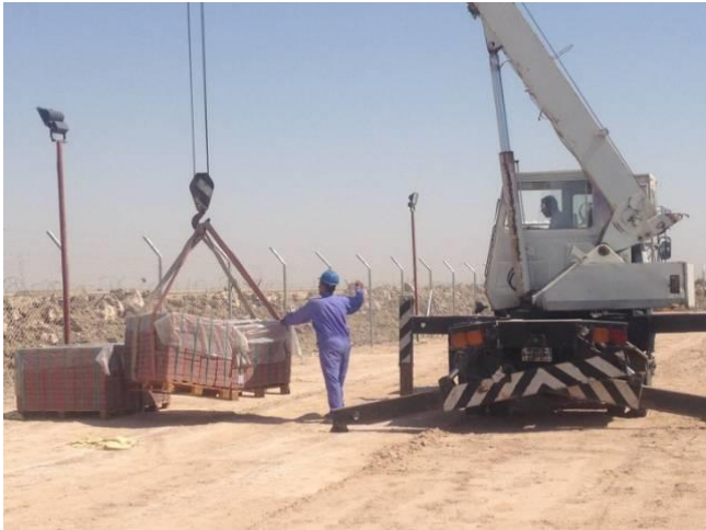
Supplying Access point control Clint: SGC Company Location: Umm Qaser Bulk storage 2006
